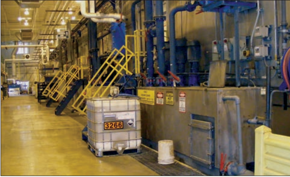
The pretreatment systems at Carrier include Suparator oil separators on the first stage and end-of-line blower systems to reduce water carryout. The cleaner is Henkel Parco ZX-1, and fluorozirconic is Henkel Bonderite NT-1.
