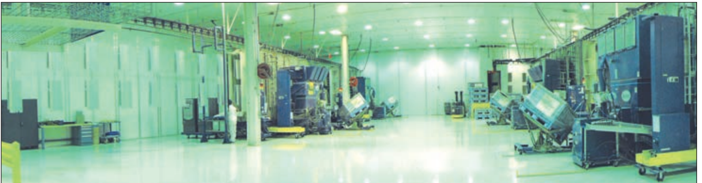
If you were to walk through Carrier's Collierville plant, you would find two separate dual line spray systems, each with a six-stage pretreatment system. There are eight cartridge-style reclaim booths with automated spray guns. The two conveyor systems are standard 4" monorail with dual drives, operating at 18 fpm.
