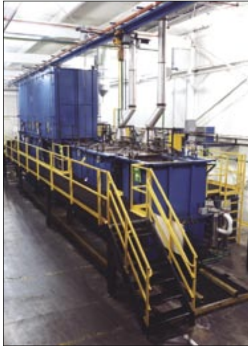
Recover process line installed at The Crown Group.
