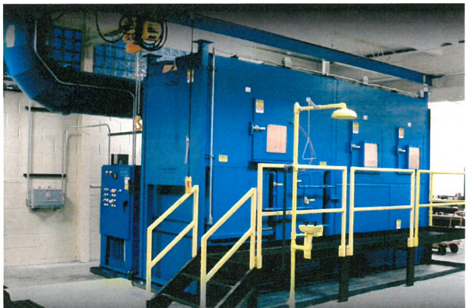
Kastech AL750 system at Carley Foundry, Blaine, MN
